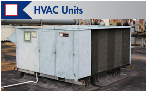
Check ductwork, housings, lines, pipes, sheet metal cabinets, gaskets, and equipment base/tie-in.
