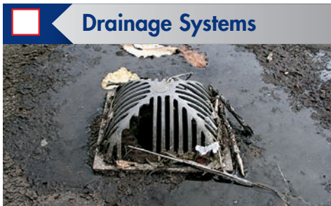
Clear all gutters, down spouts, and scuppers; clean out drains; check strainers and clamping rings.
