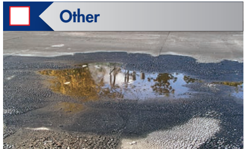
Check for oil deposits, surface contamination, soft areas, vandalism, and ponding water.
